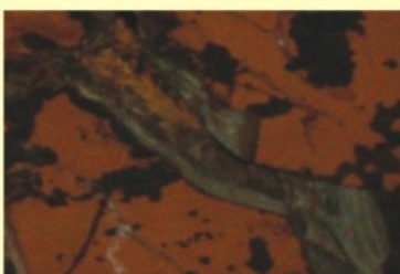
Cracks on the tunnel
